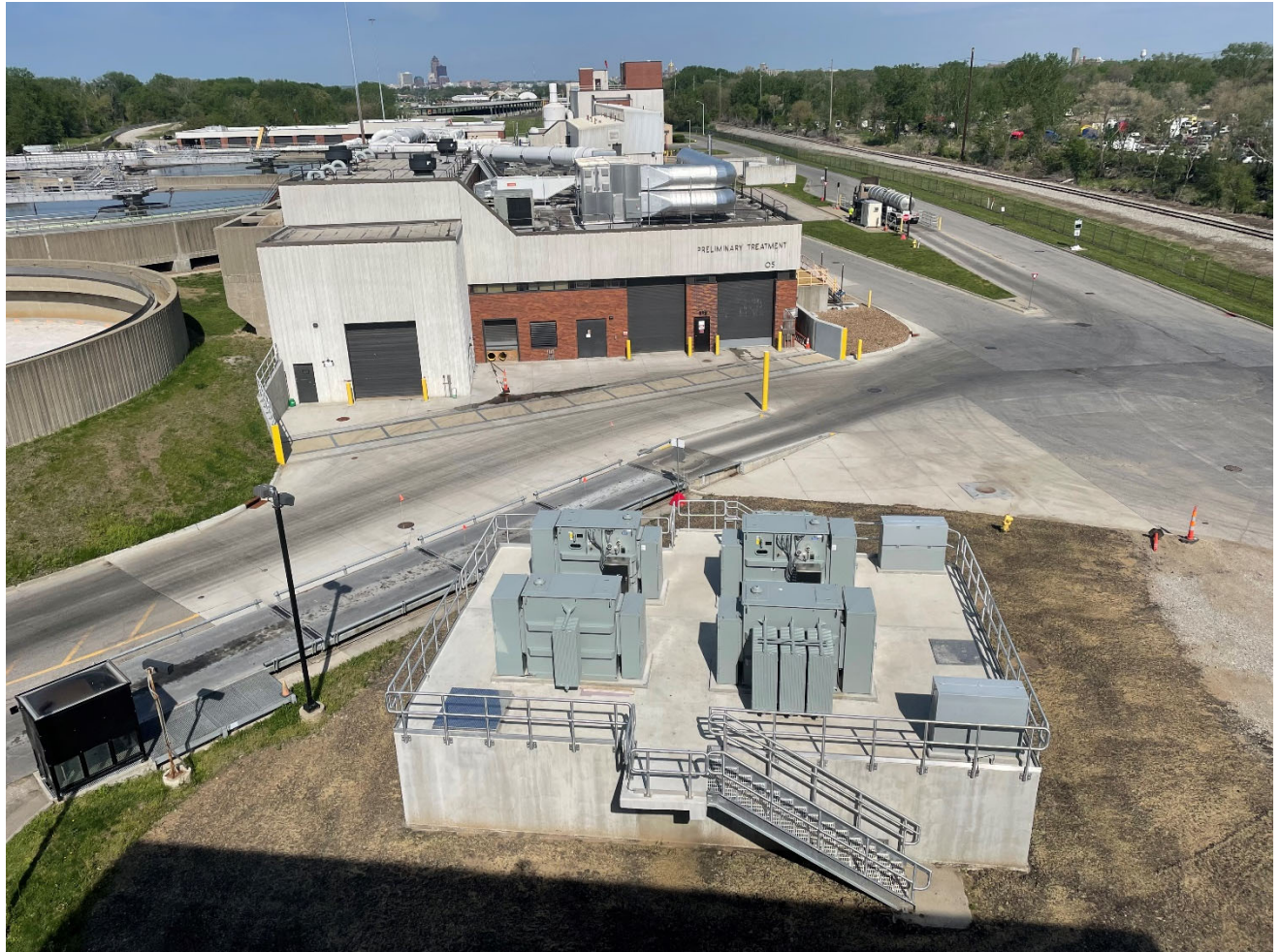
Figure 2: Elevated Electrical Transformers the Serve Main Pump Building and floodwall protecting Preliminary Treatment Building in background
