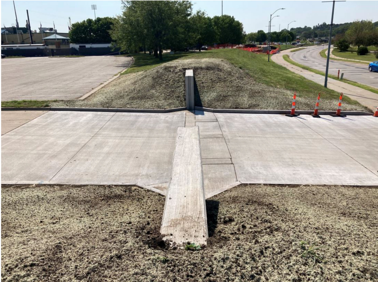
New stop log closure installed as part of Phase A of the Levee Alterations at the parking lot access at Principal Park.
