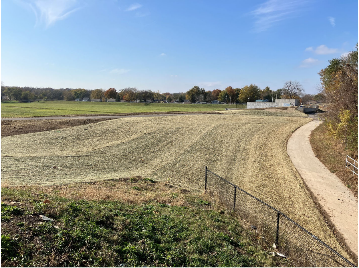
DSM Levee Alt Phase C, south side of Des Moines River between SE 14 th Street & Jackson Pump Station
