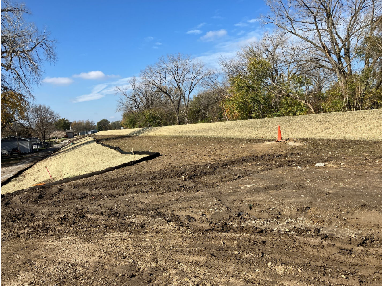
DSM Levee Alt Phase C, south side between SE 6 th Street & SE 9 th Street
