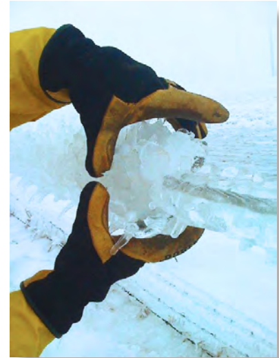
Ice covering a power line.
