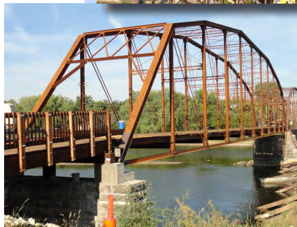
Top: Sutliff Bridge during construction in August 2012. Below: The same bridge in September.
