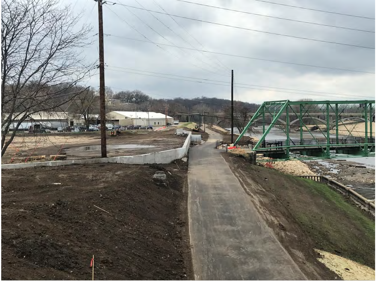
DSM Levee Alt Phase B, SW 3 rd Street - SW 7 th Street, south side floodwall
