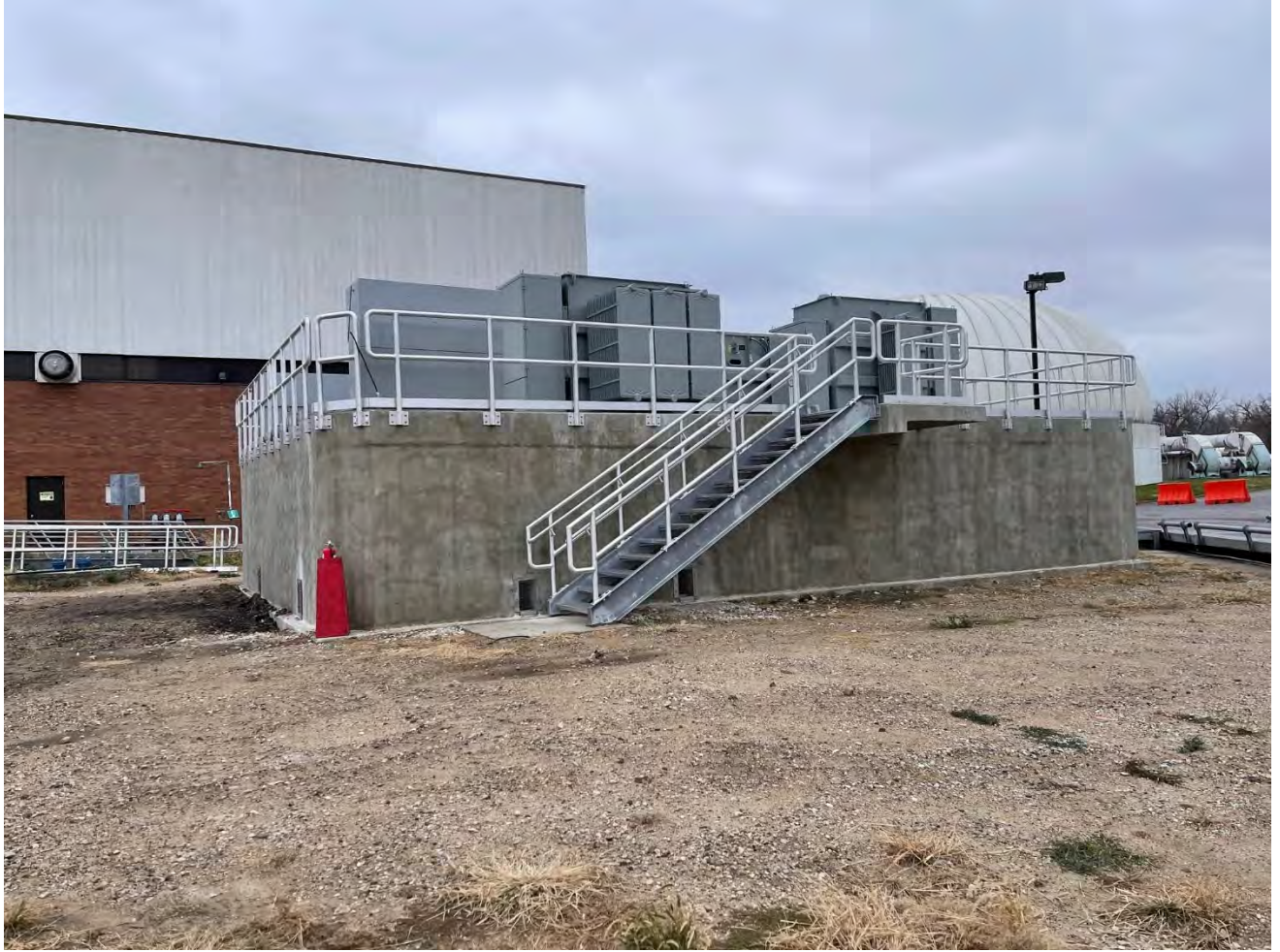
Figure 2: Elevated Electrical Transformers the Serve Main Pump Building
