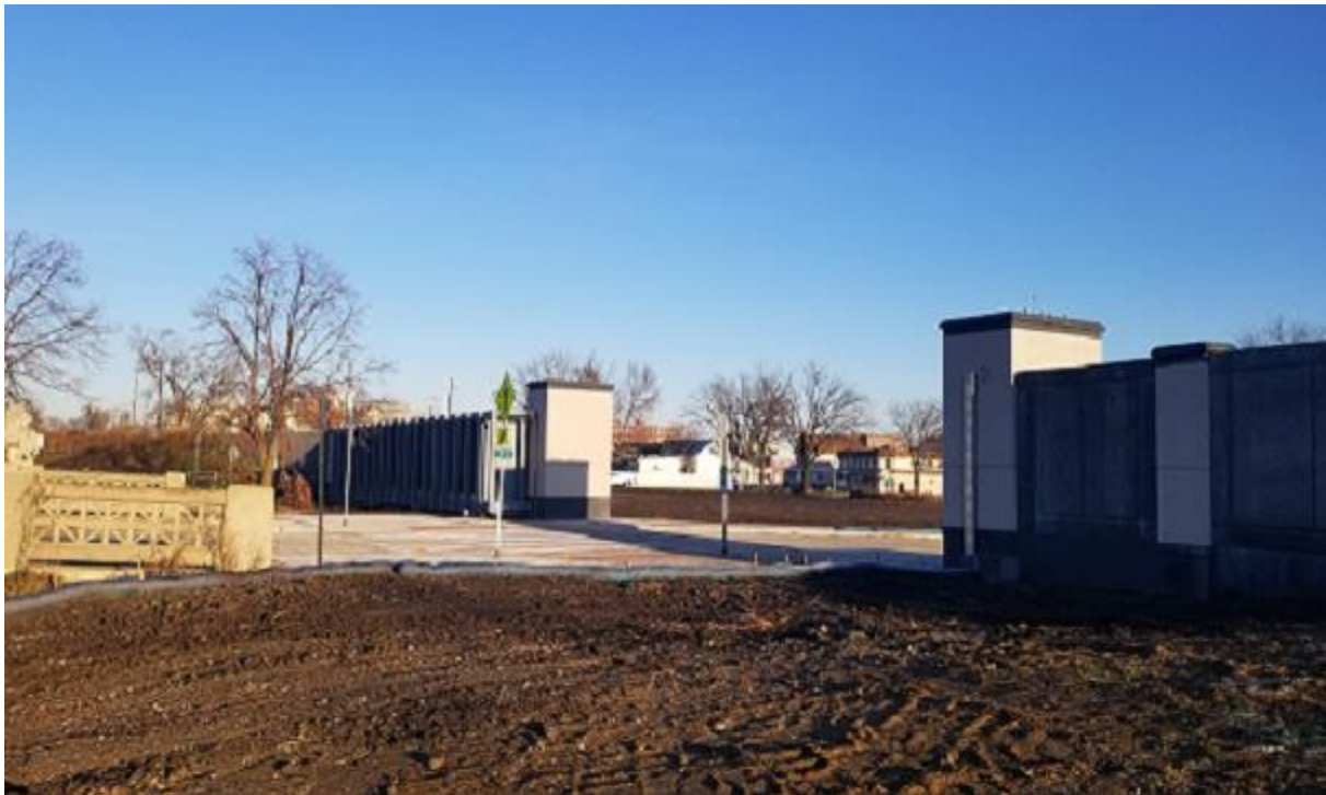
16 th Avenue SE Roller Flood Gate – November 2020
